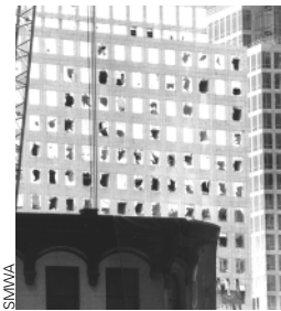
Windows blown out
