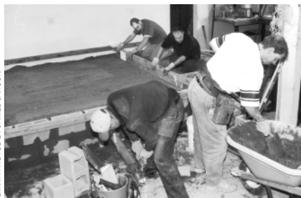
THE LAY ORDER OF ST. MICHAEL building a platform for our 22-foot web press.
